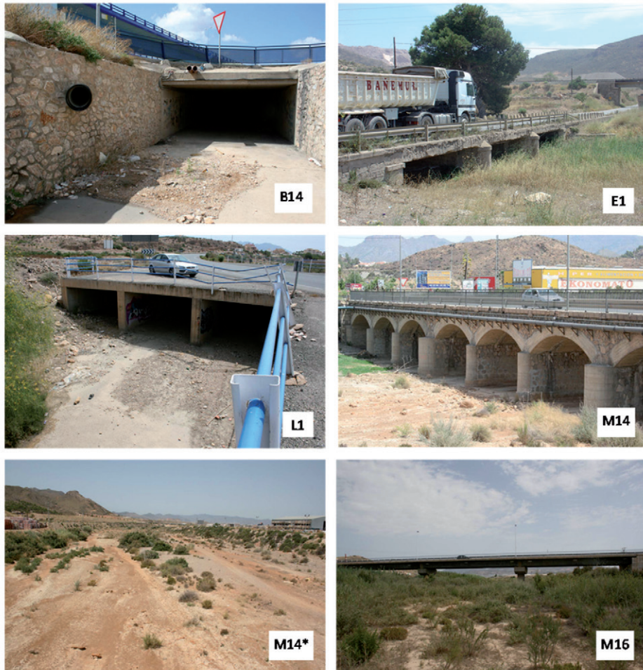
Figure 3. Pontoon in point B14: road crossing the connecting channel between the Dolores Rambla and the Benipila Rambla . Point E1: the Escombreras Rambla intersecting with Mu-320 (local tertiary road). Point L1: crossing of N-332-1 road over the Lorentes Rambla saved by pontoons. Point M14: road N-332-1 over the Moreras Rambla next to Mazarrón (lower reach). Point M14*: sandy loam bed upstream from the M14 bridge over the Moreras Rambla . Point M16: the intersection of the Moreras Rambla with D-6 (local tertiary road) which links Mazarrón Port with Bolnuevo (Águilas).
