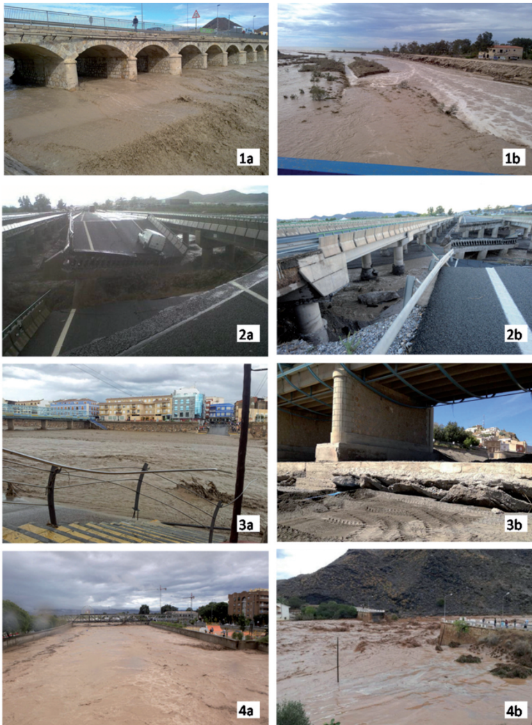
Figure 5. Flooding by ephemeral channels on September 28th, 2012, affecting bridge crossings in South East Spain. Scour holes downstream of crossings M14 (1a) and M16 (1b); Failure of the bridge due to scour at their foundations on the A-7 over the Béjar Rambla (2a and 2b); Nogalte Rambla at the point where it passes through Puerto Lumbreras before (3a) and after the flood (3b); Guadalentín Rambla at its pass through Lorca (4a); Old bridge destroyed by flooding in Lobos Rambla (4b).
